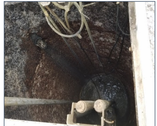
Figure 1: Lift Station A
