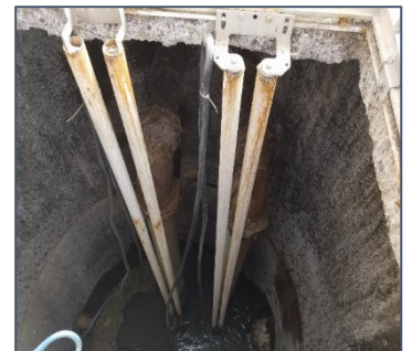
Figure 3: Lift Station E
