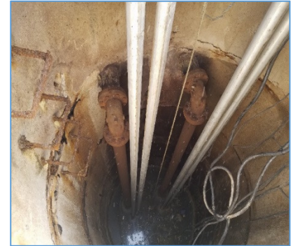
Figure 2: Lift Station C
